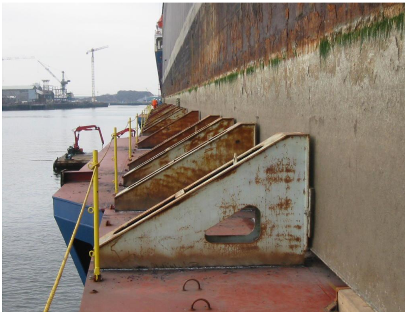
Steel brackets securing the floating dry dock
